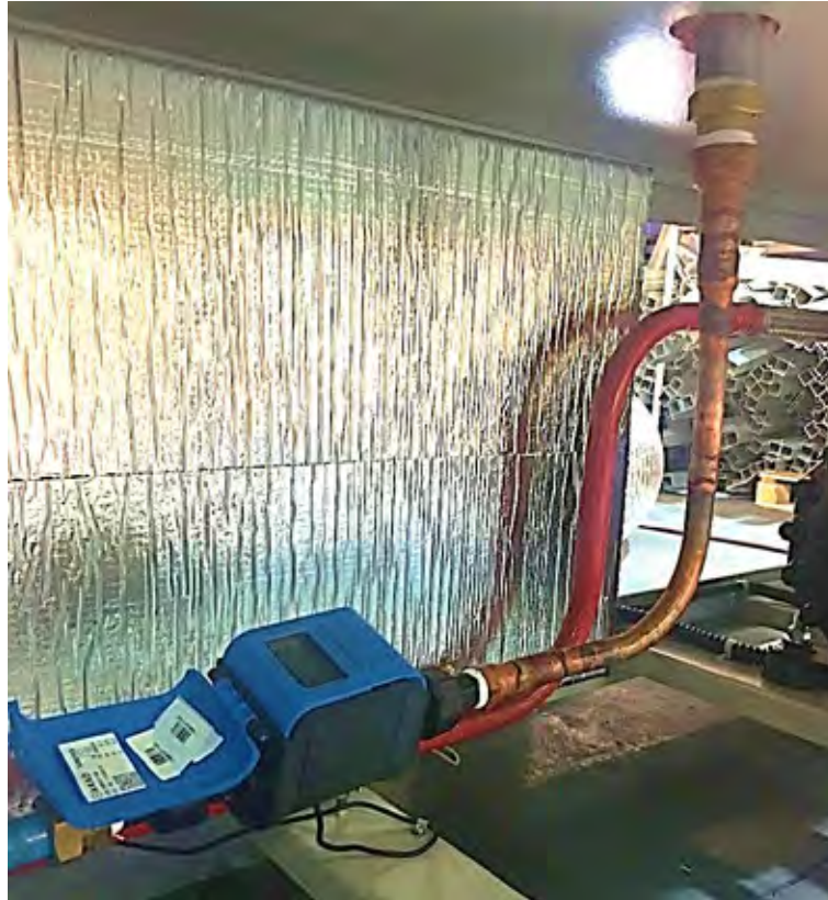
Figure 17. Installed water meter
