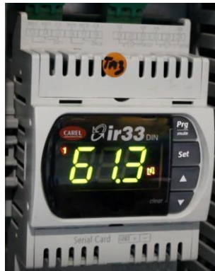
Figure 9-6. Temperature valve controller
