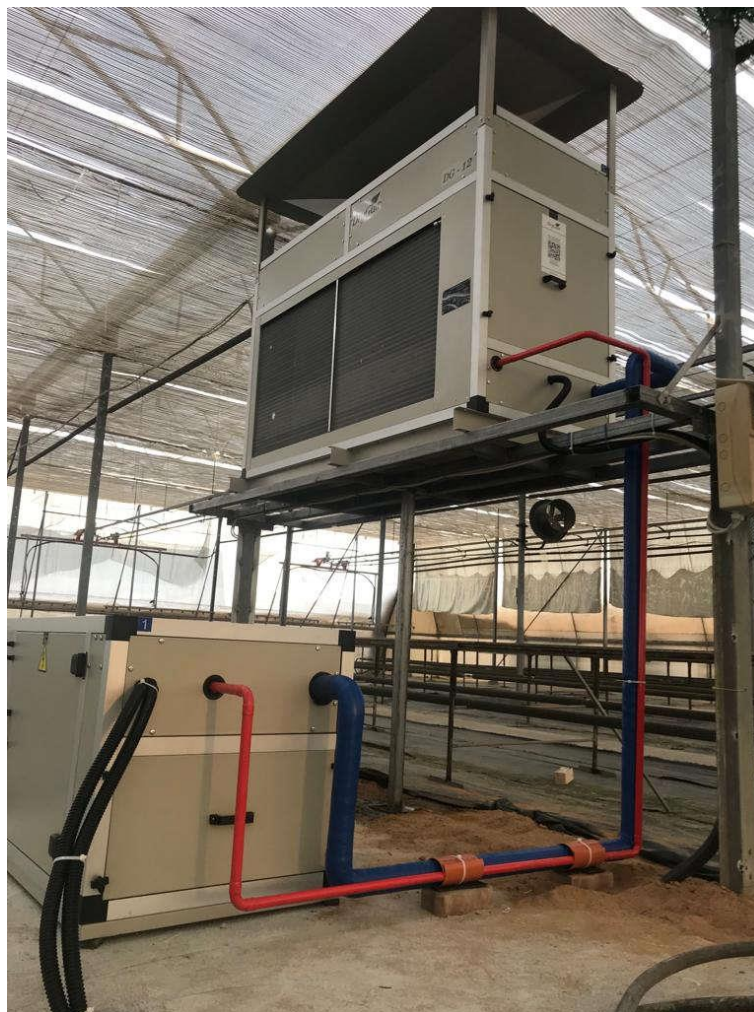
Figure 9-7. DryGair split unit
